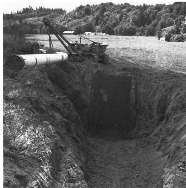
Construction of Northwest Natural Gas Company feeder pipeline just east of Mist.
