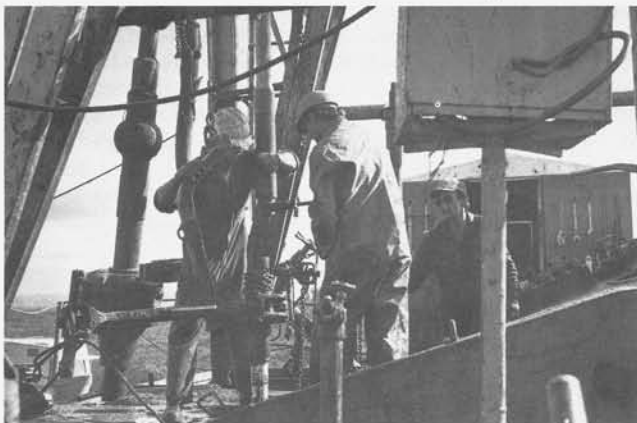
Driller and roughnecks running drill pipe into Columbia County 23-35, Mist Gas Field. The well was later plugged and abandoned.
